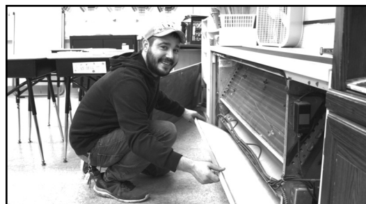
Cody Luchenbill is shown changing a classroom heating unit ventilator at Corunna Middle School.
